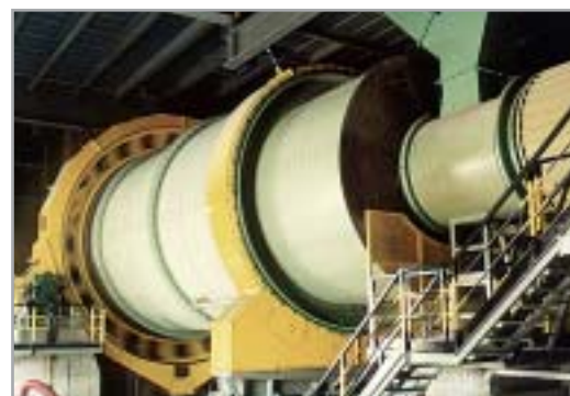
Raw mill \varnothing 5.4 x 11 m with a pre-drying chamber
